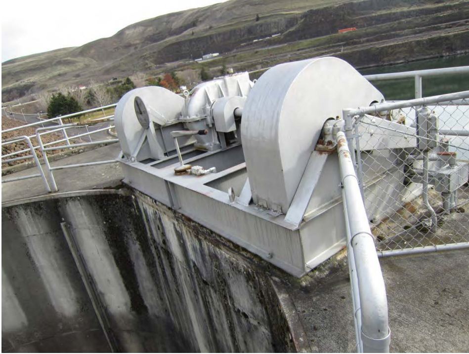
Figure D-3. Electrical Equipment, Fishlock Entrance Gate
