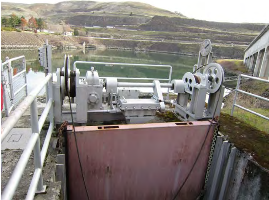
Figure D-2. Electrical Equipment, Fishlock Approach Channel
