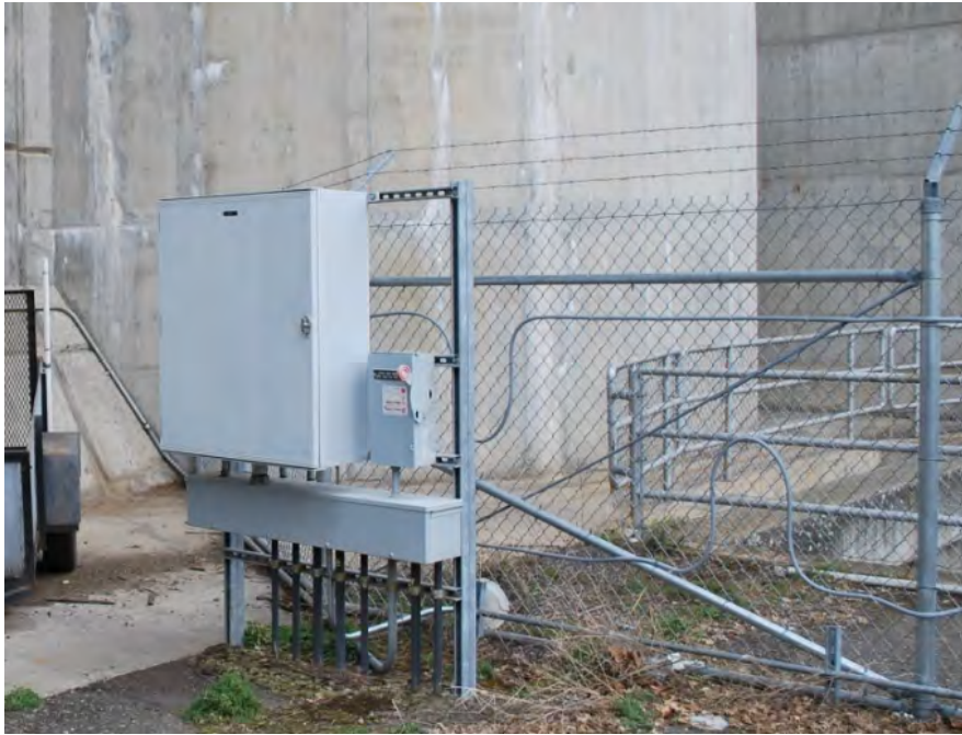
Figure D-1. Electrical Equipment near Fishlock
