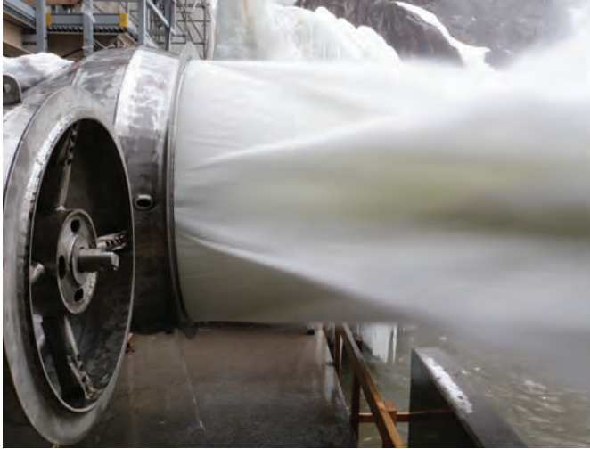
Williams Fork Dam, Colorado, USA—Three Ring Jet Valves (12", 20", and 36") and three Rotovalve® Cone Valves (16", 24", and 42").
